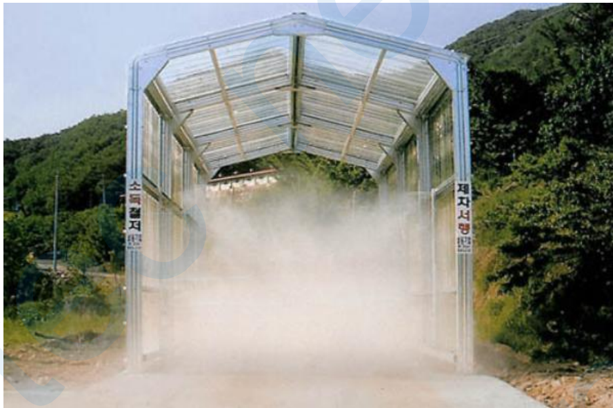
Disinfection channel for trucks and buses
