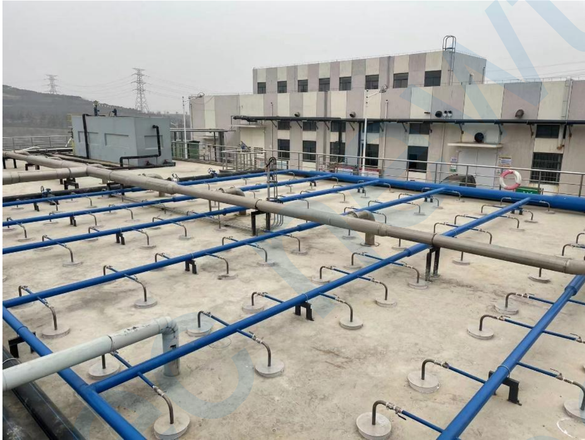
VAS aerators: 140 sets
