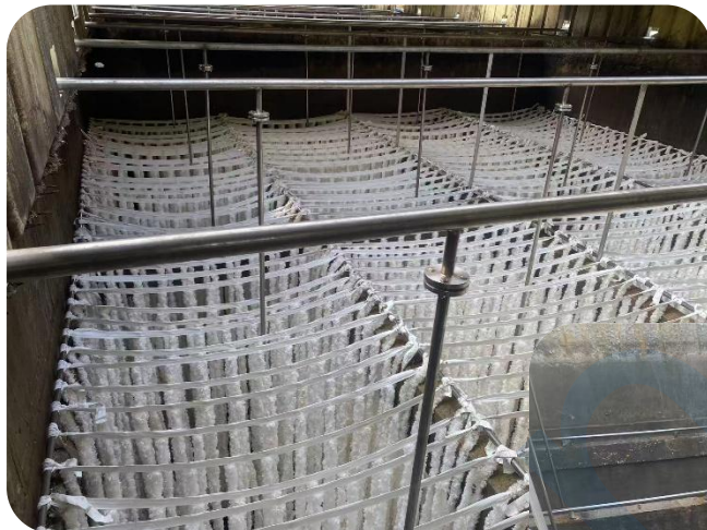
Hydrolysis acidification Tank
