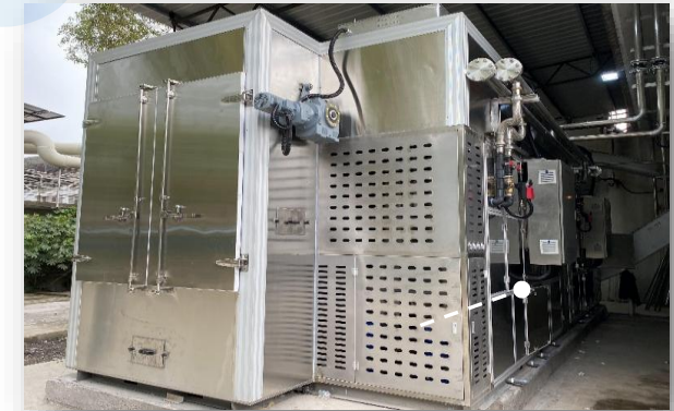
Heat pump compressor installed in a separate compartment
